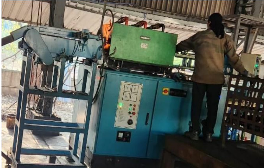
200 KW INDUCTION BILLET HEATING
